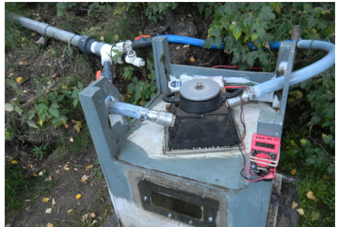
Rapids Research new water power system at main camp, 2012
